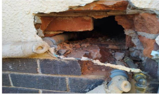
Photo Caption: Area where the pipe burst
