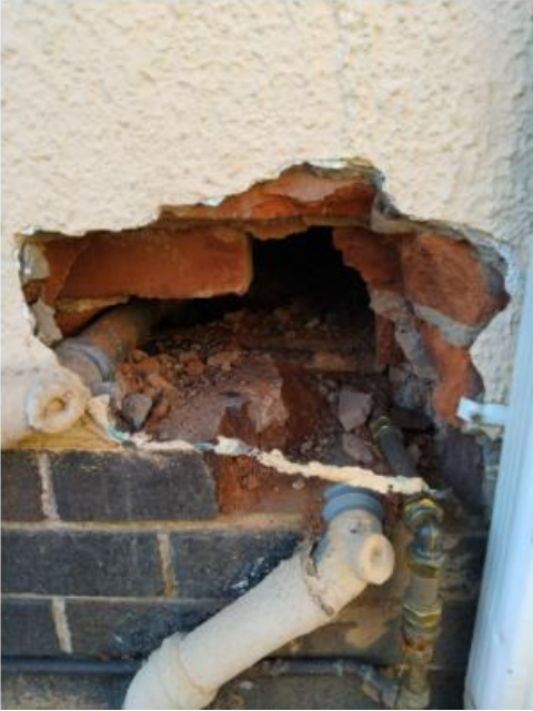
Photo Caption: Area where the pipe burst
